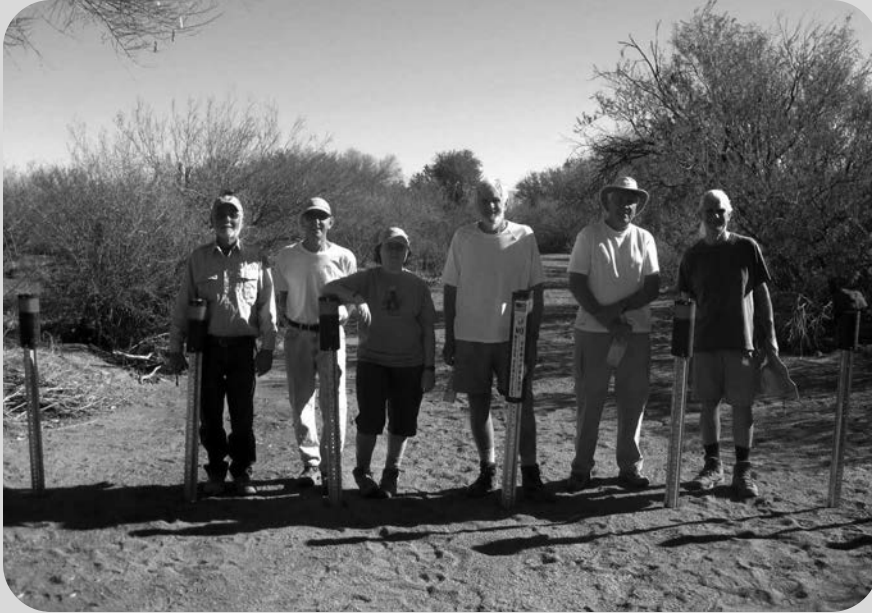
Volunteers install barriers to keep people from driving in washes of Ironwood Forest National Monument. Left to right, Al Mezzano (Bureau of Land Management Park Ranger), Ed Nigl, Kathy Church, Gary Borax, Richard Muzzy, and Jim Avramis. Photo courtesy Jim Avramis.
